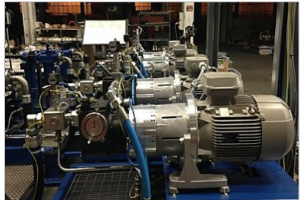
Application on high pressure machine for polyurethane
